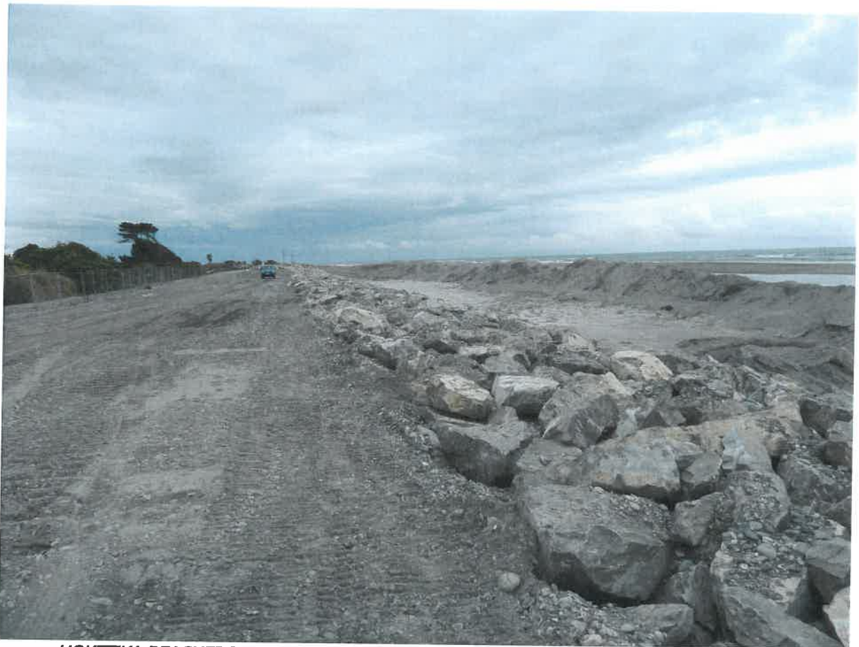
HOKITIKA BEACHFRONT SEAWALL – 27 SEPTEMBER 2013 Top View Looking Southwards Showing completed rockwork and sand bund
